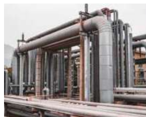
Natural Gas Station
